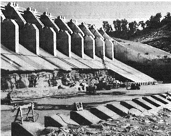
a) Severe damage to spillway
