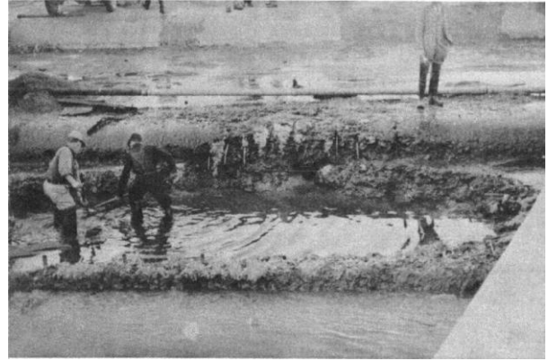
b) Damage to Positive Steps and Floor
