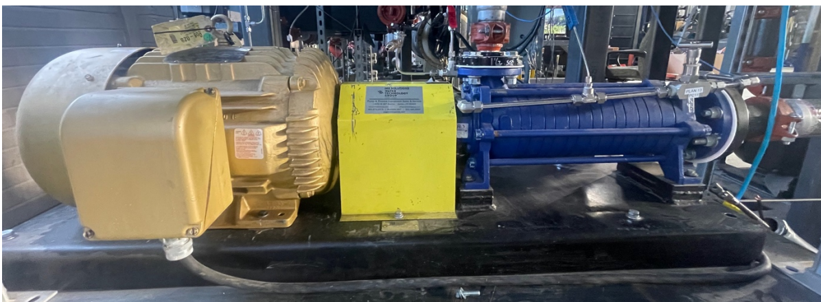
Figure 3-19: SERO SRZS 446 power cycle pump installed in the hybrid ORVC test facility.
