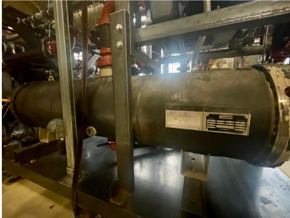
Figure 3-17: The shell and tube spray evaporator installed in the test facility.
