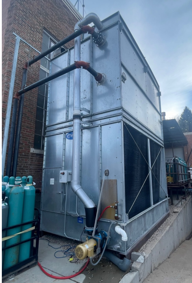
Figure 3-24: Evaporative cooling tower installed outside of the Powerhouse Energy Campus.
