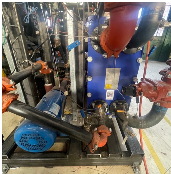
Figure 3-26: Evaporator loop equipment including pump and plate heat exchanger as installed in the test facility.
