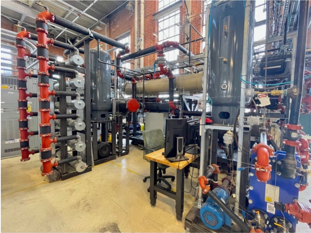
Figure 3-4: Overview photo of the hybrid ORVC test facility as configured for this research.
