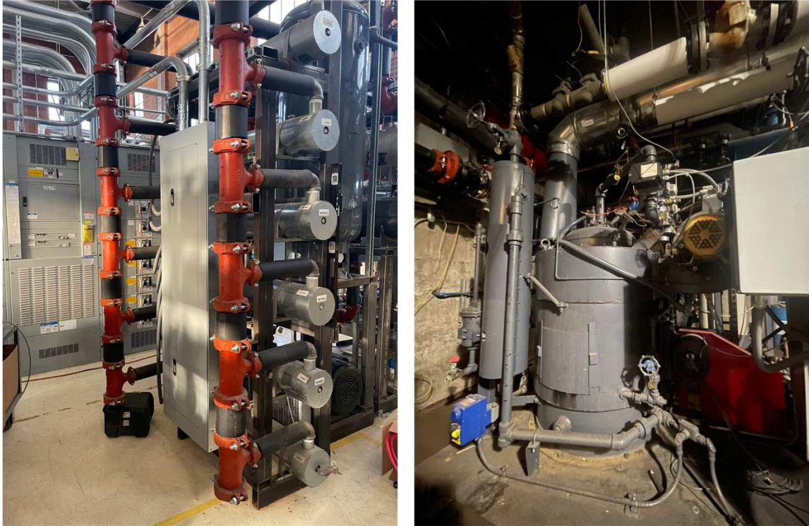
Figure 3-22: The six circulation heaters (left) and natural gas steam generator (right) that provided heat to the heat supply circuit.
