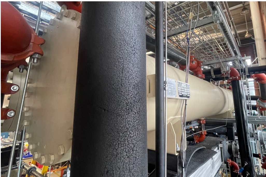
Figure 3-16: Photo of the cooling cycle condenser installed in the hybrid ORVC test facility.
