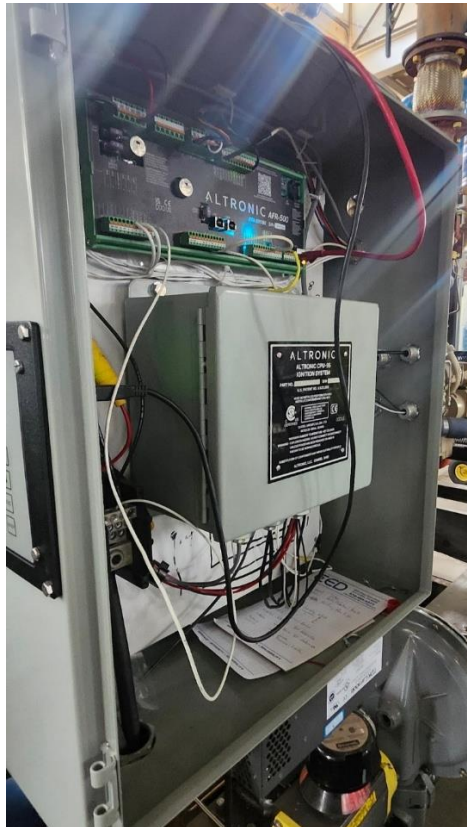
Figure 7: Altronic Controls Panel
