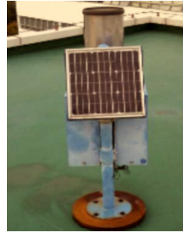
(b) rainfall observation equipment
