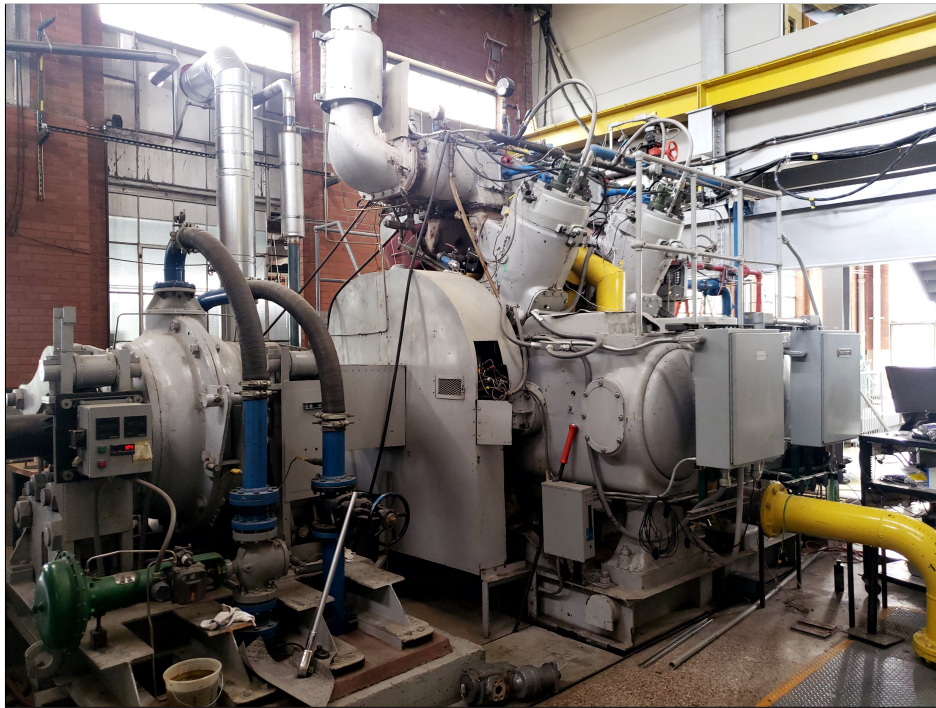
Figure 2.1: GMV-4TF engine housed at CSU's Energy Campus inside the Powerhouse.
