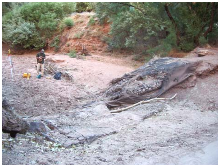
Figure 3.10 In-channel structure immediately below knickzone in longitudinal profile at 13.0 km that partially functions as a grade control. Erosion is evident at top center of structure. Differences in bed elevation immediately upstream and downstream from structure is 0.42 m.
