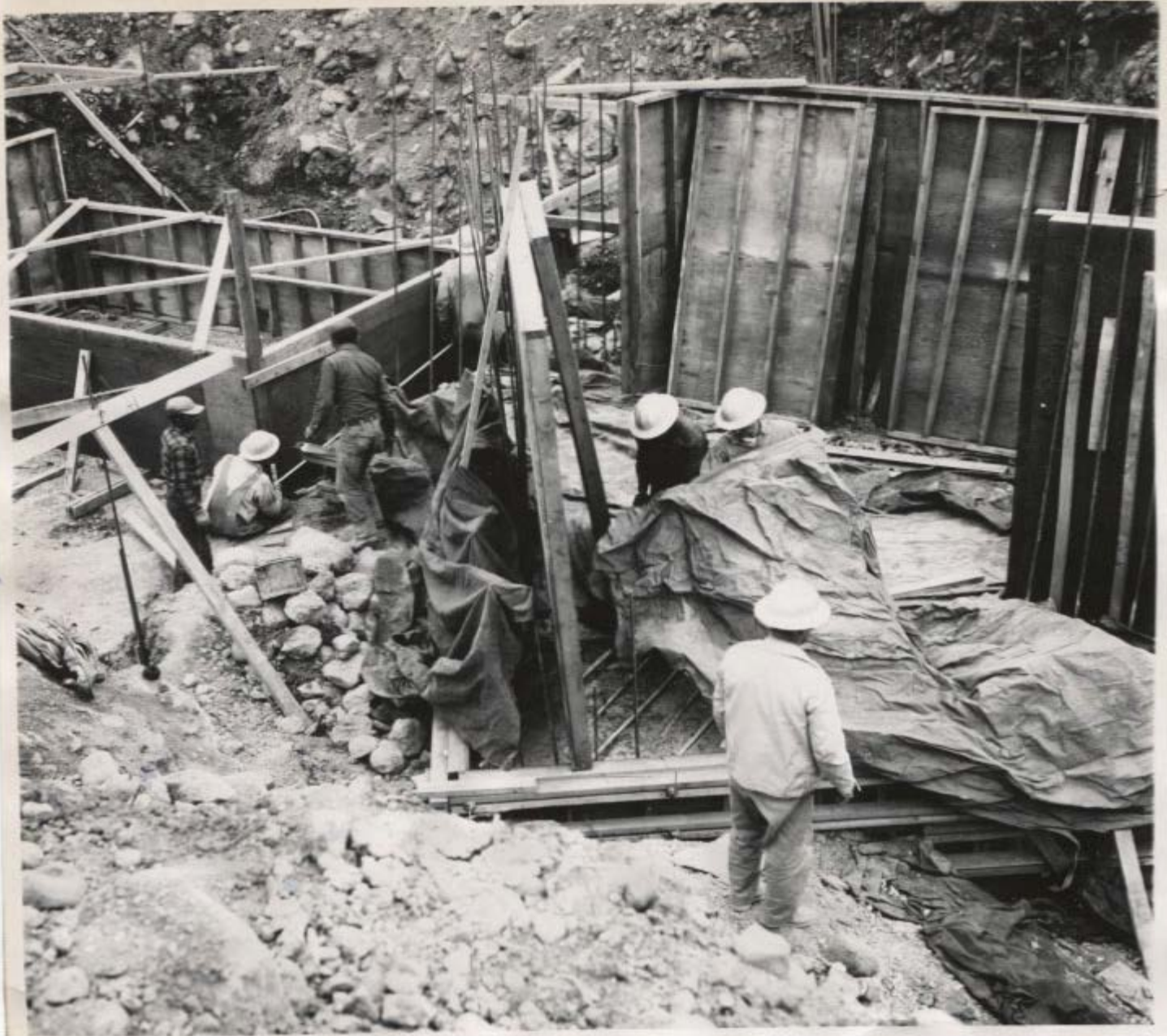
PLANT WORK — Forms for the substructure of the Upper Molina Power plant of the hamlet of Molina in the Plateau Valley go into place as Coll-
