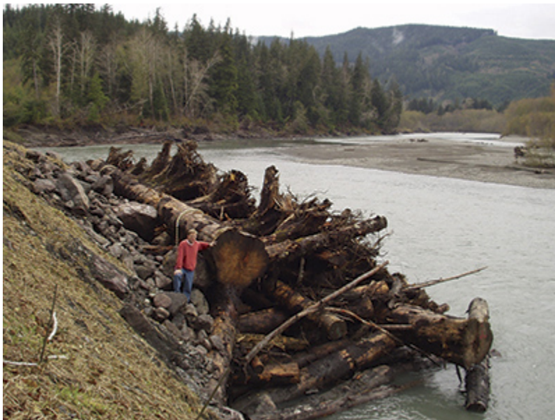
Figure 4. An example of a large engineered logjam built by the Washington State Department of Transportation on the bank of the Hoh River along U.S. Highway 101.
