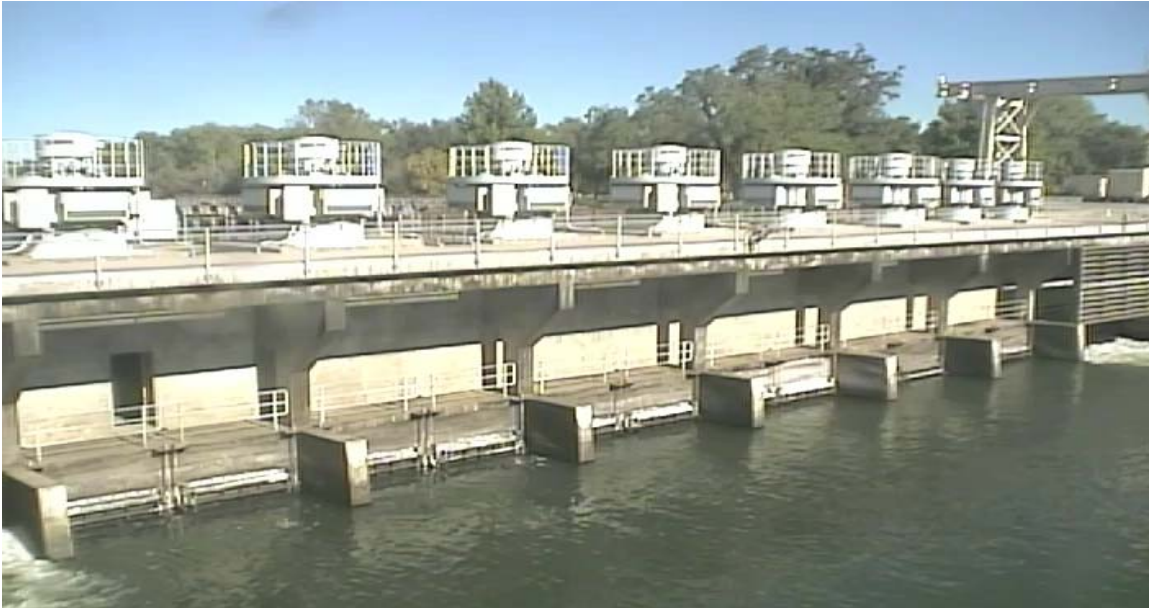
Figure 2. GCID's main pump station, located on the Sacramento River, has the capability of pumping 3,000 cubic feet per second (cfs). SCADA allows canal operators to make pump changes remotely, monitor water elevations, and measure the water quality entering the District's main canal.
