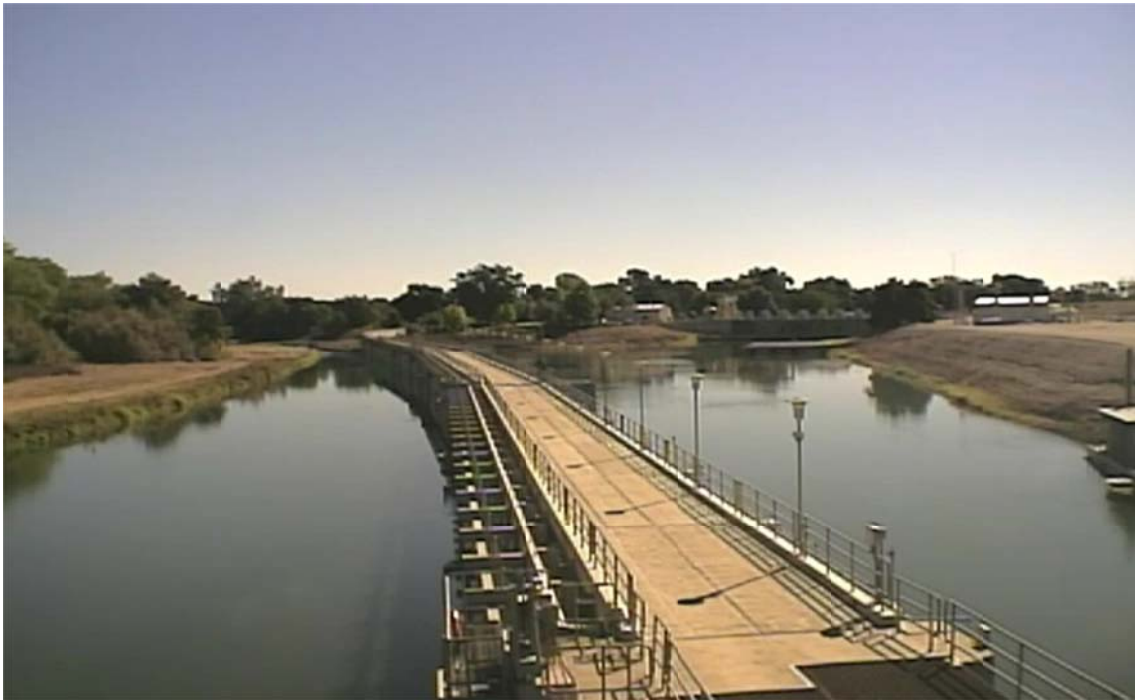
Figure 1. SCADA allows GCID to monitor the activities of its 1,100-foot long fish screen. The pump station is located directly behind the fish screens.
