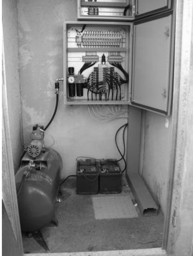
Figure 3- Interior of the hut. Motor, compressor, tank, batteries, etc.
