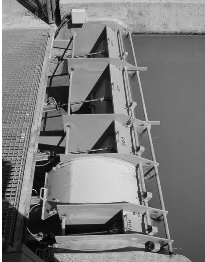
Figure 6. Sector modules, with horizontal pneumatic cylinders.
