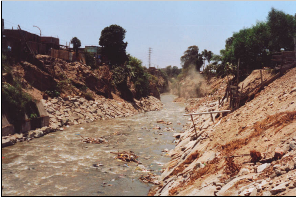
Figure 5. This photograph shows the rock ramp downstream of the Dueñas bridge. This picture was taken from the right bank of the river.
