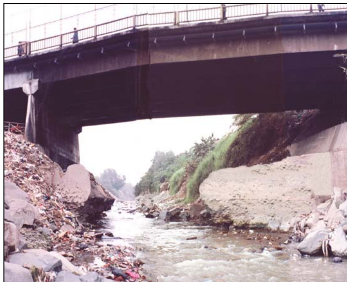
Figure 2. View showing the bed level in 2001. Notice that the river flows underneath one opening. Also notice scour in the right bank (left) and leftovers of a remedial work.
