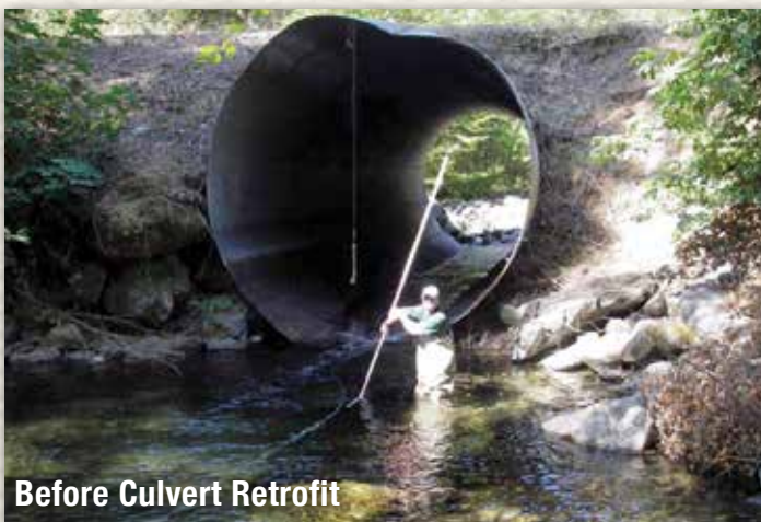
Bridge culvert impeding fish passage in Fort Goff Creek, Klamath National Forest, California. Photo courtesy of USFS.
