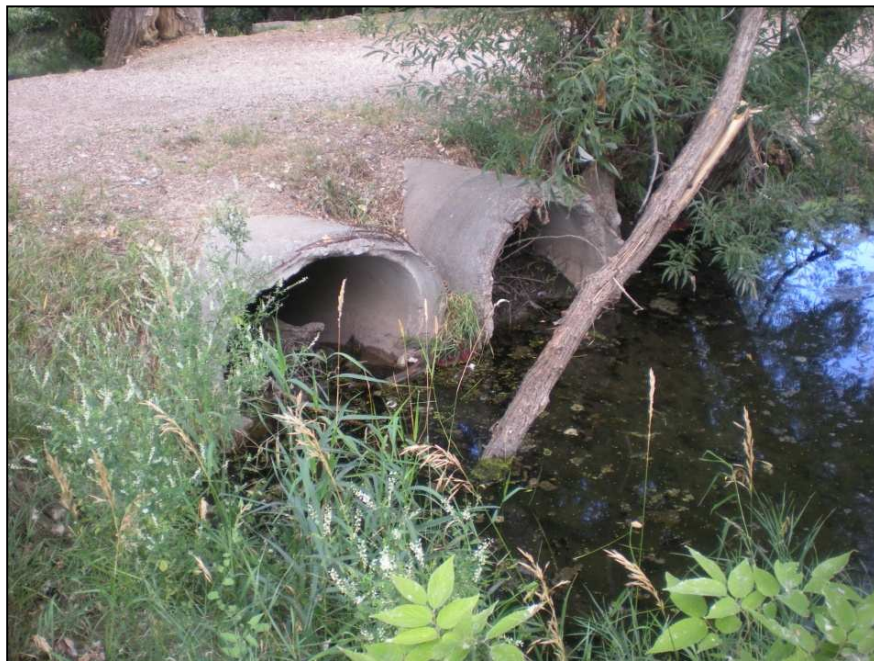
Figure 3.6. The Howes Street Basin wetland outlet culverts to the Poudre River
