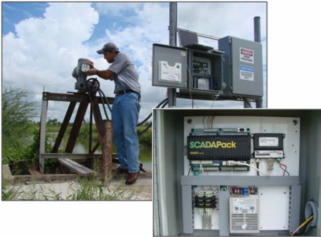
Figure 3. The Remote Terminal Unit (RTU), which consists of PLC, radio, power converter, fuses and terminals and actuator at the Emergency Gate site.
