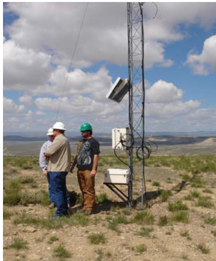
Figure 2. Selecting the best repeater site and adding additional hardware takes time and study to ensure the best results.
