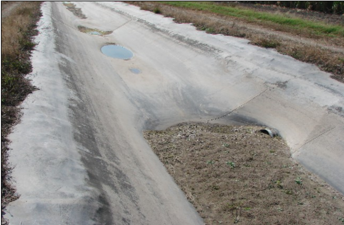
Figure 3. Aquatic vegetation and sedimentation clogging a farm outlet pipe
