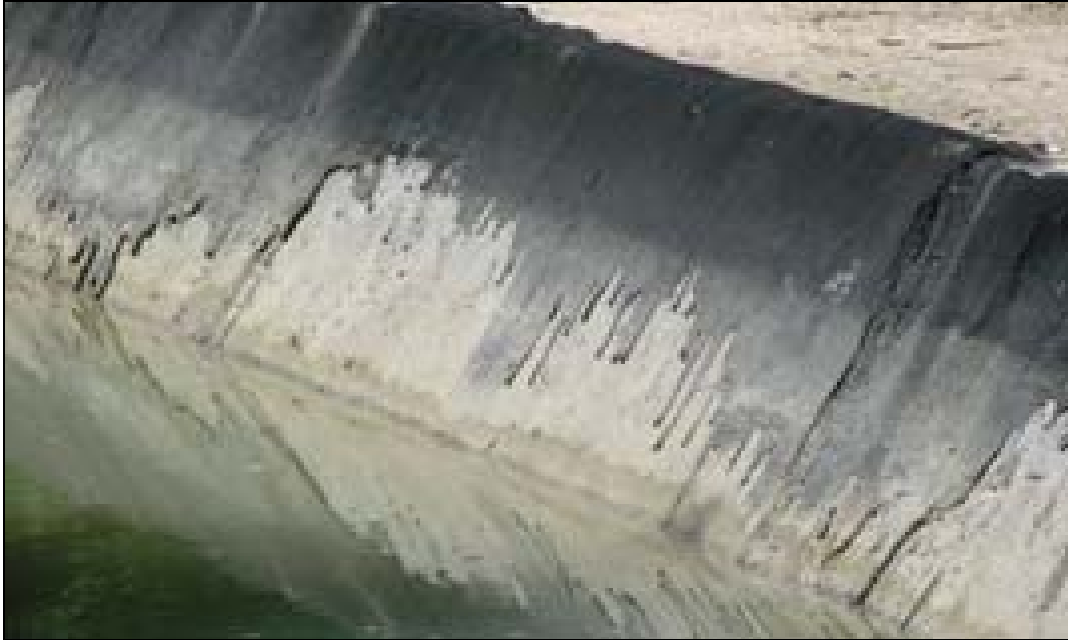
Figure 9. Residue left from a deteriorated polyurethane liner
