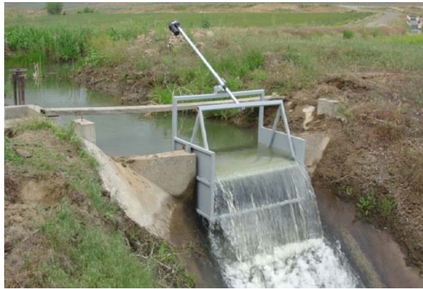
Figure 10. Self-constructed overshot gate in eastern Oregon.
