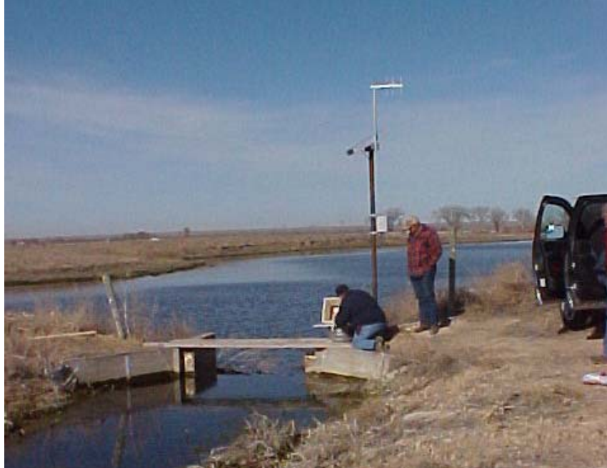
Figure 2. 2005 Installation at the SPDC Sandhill Pond Entrance
