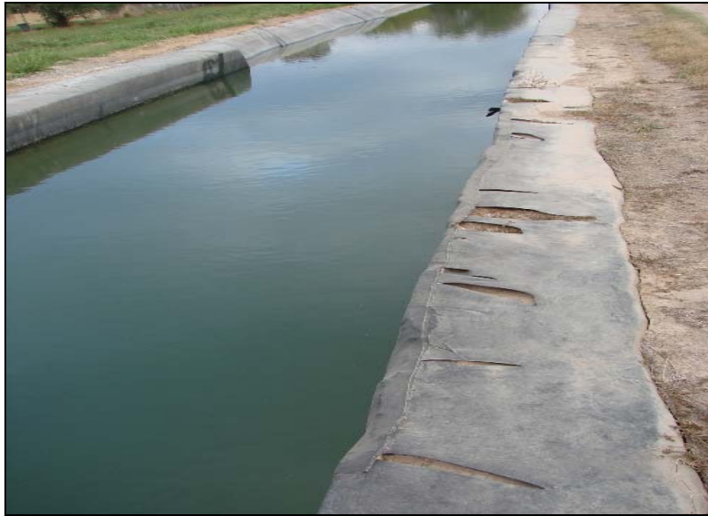
Figure 6. Cuts/tears in a rubber liner
