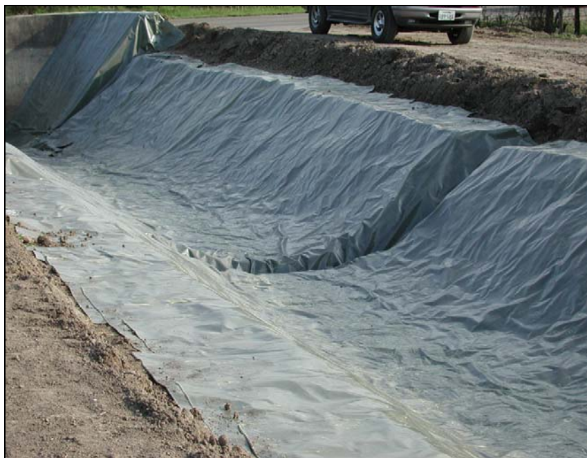
Figure 11. Canal liner installed too low on the levee
