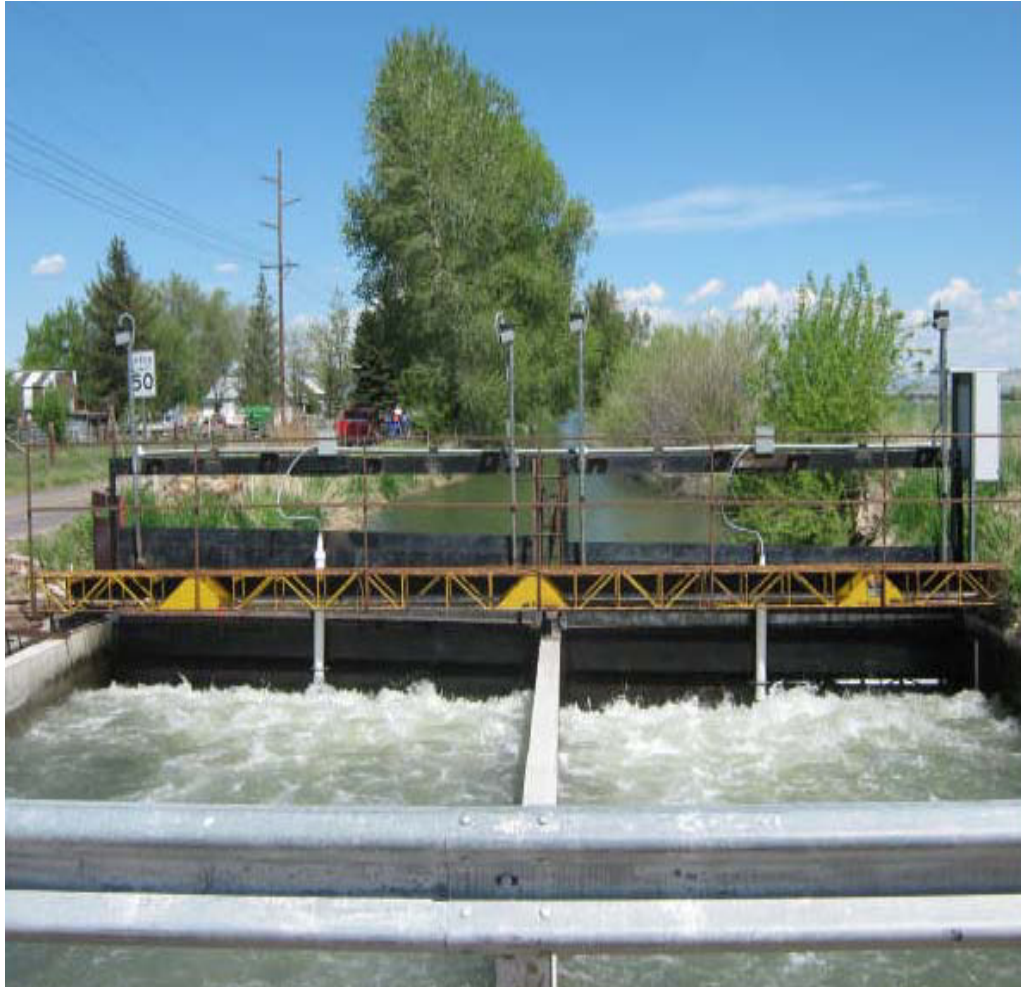
Figure 3. Side by side large slide gates with two linear actuators on each gate
