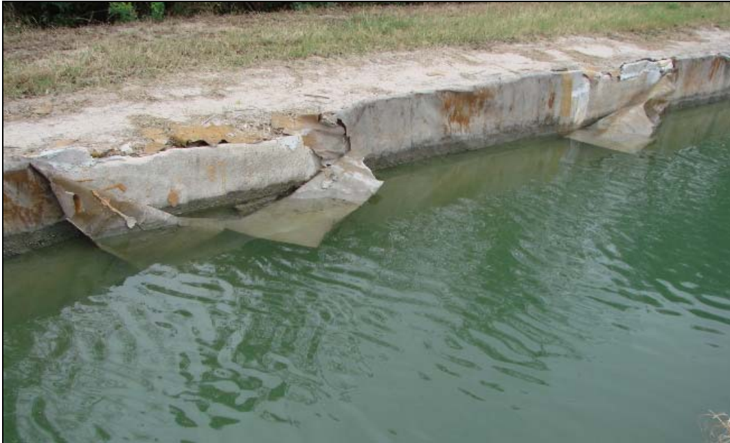
Figure 8. Polyurethane liner is shown hanging off the canal wall.
