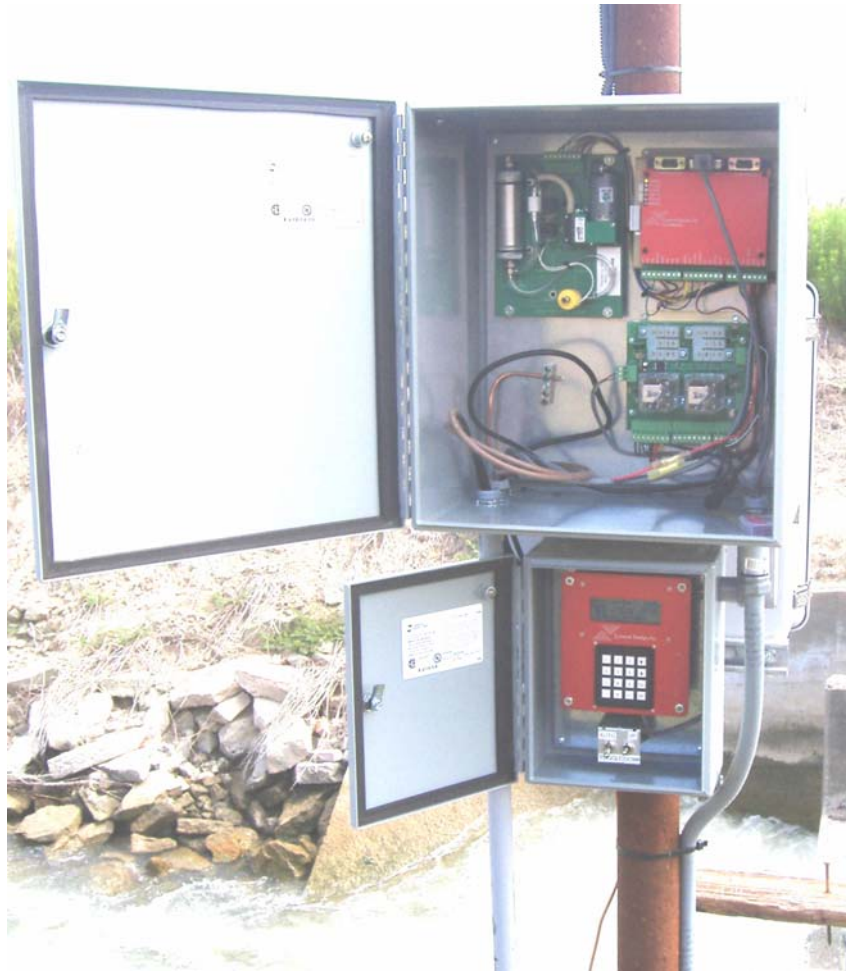
Figure 6. Control Components (upper enclosure) and User-Interface Components (lower enclosure)
