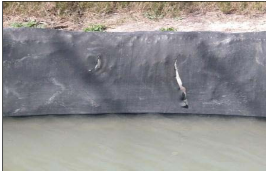
Figure 14. Vertical cut or tear on canal side wall caused unintentionally
