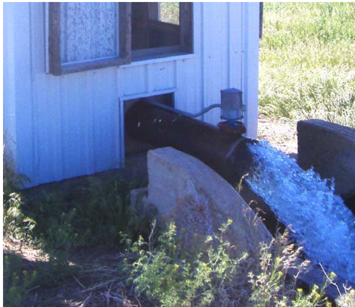
Figure 5. A Pulse Output Module Installed on a McCrometer Meter at a J & E Well
