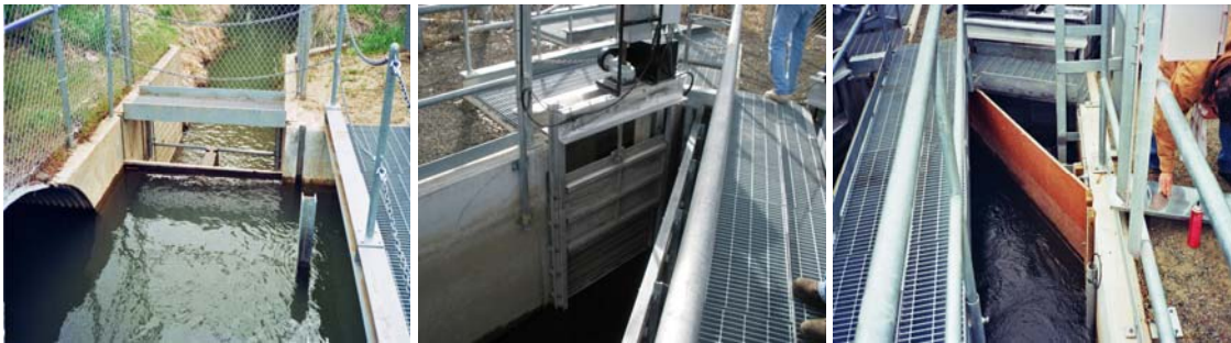
Figure 2. Packwood diversion structure showing passive operational spill, automated operational spill, submerged orifice, and automated gate in front of paddlewheel
