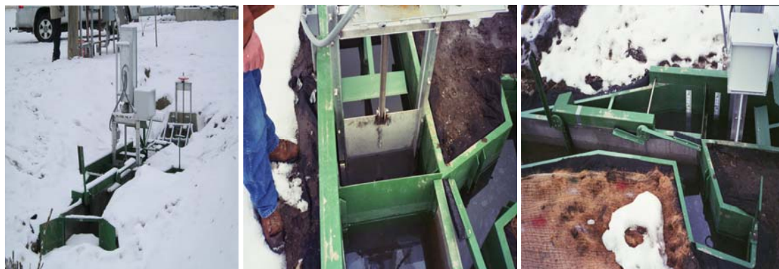
Figure 4. Nisbet diversion showing the completed structure, automated regulating gate after the submerged orifice, flat plate fish screen and location of staff gauges for determining head differential between forebay and orifice bay.
