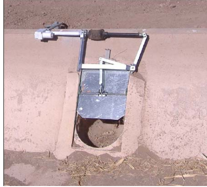
Figure 7. Linear actuator on turnout gate at the Imperial Irrigation District automated surface irrigation demonstration site
