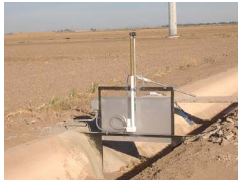
Figure 9. Linear actuator on check gate at Imperial Irrigation District automated surface irrigation demonstration site
