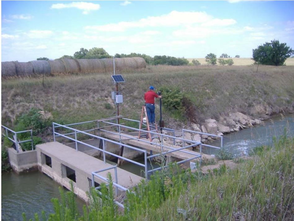
Figure 4. Reclamation Engineer Clinton Powell Making Wiring Connections on the Linear Actuator at the Nebraska Bostwick 20.2 Check
