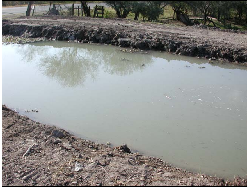
Figure 12. Water level higher than the canal liner installed
