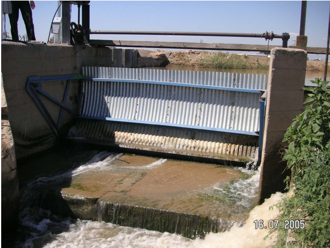
Figure 3. Retrofitted Automation – New Cache La Poudre, Colorado, USA
