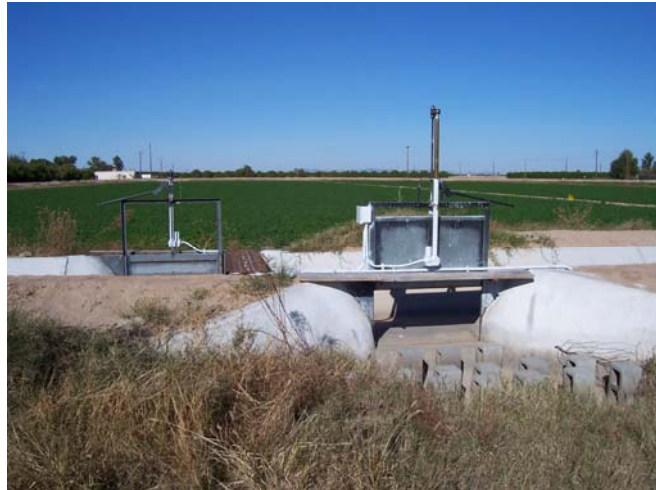
Figure 6. Alfalfa field turnout gates
