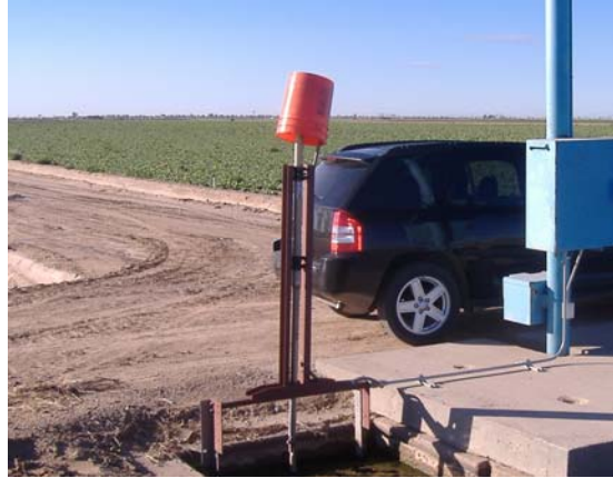
Figure 12. Linear actuator on a slide gate with an inverted bucket installed over the motor and gearbox to prevent moisture damage.
