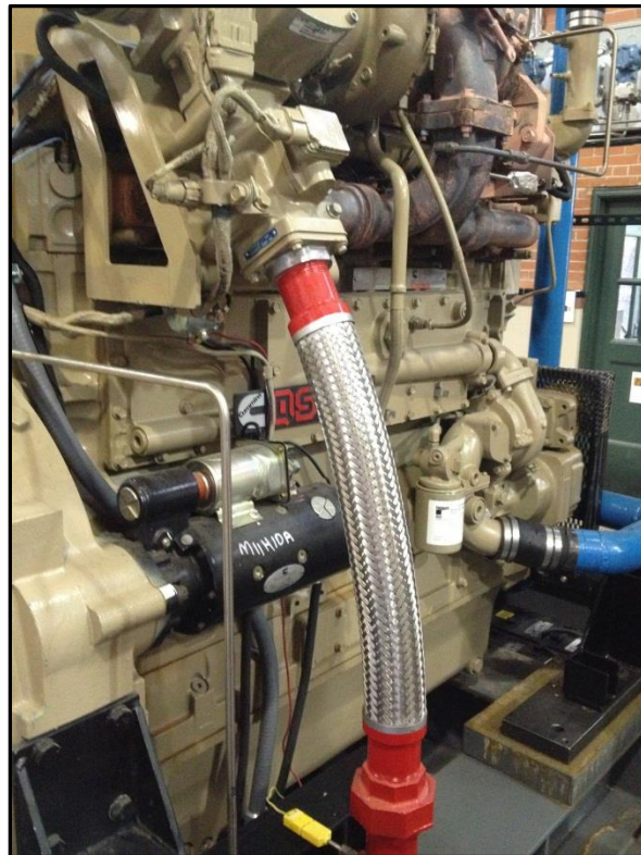
Figure 12. Natural Gas Flex Line.
