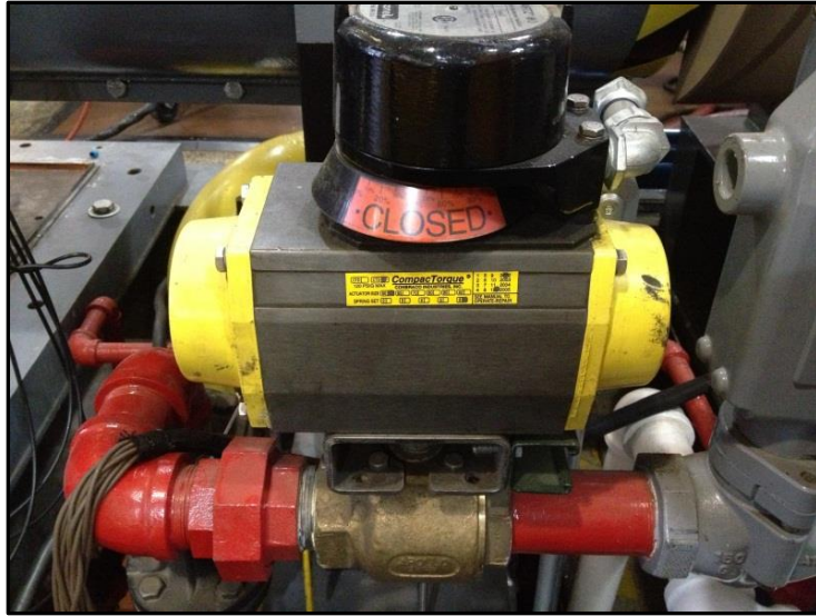
Figure 11. Natural Gas Block Valve.
