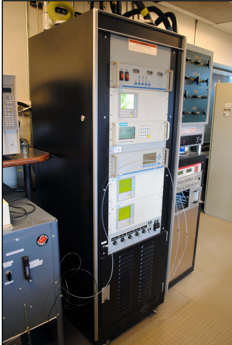
Figure 22. 5-Gas analyzer rack with a combination of Rosemount and Siemens instruments.
