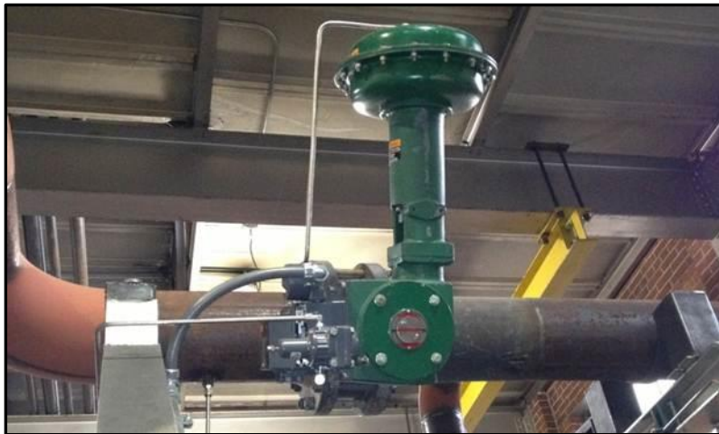
Figure 13. Exhaust Back Pressure Valve.
