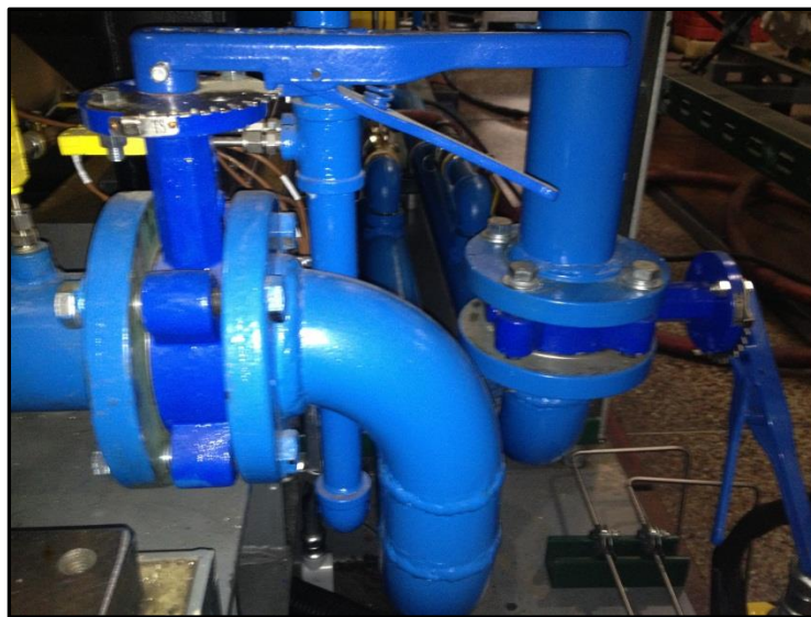
Figure 6. Jacket Water Flange Connections.
