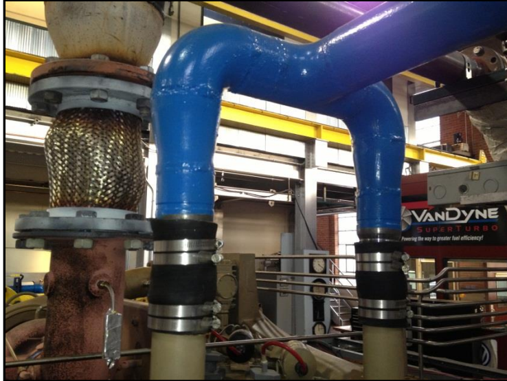
Figure 7. Engine Coolant Return Connections.
