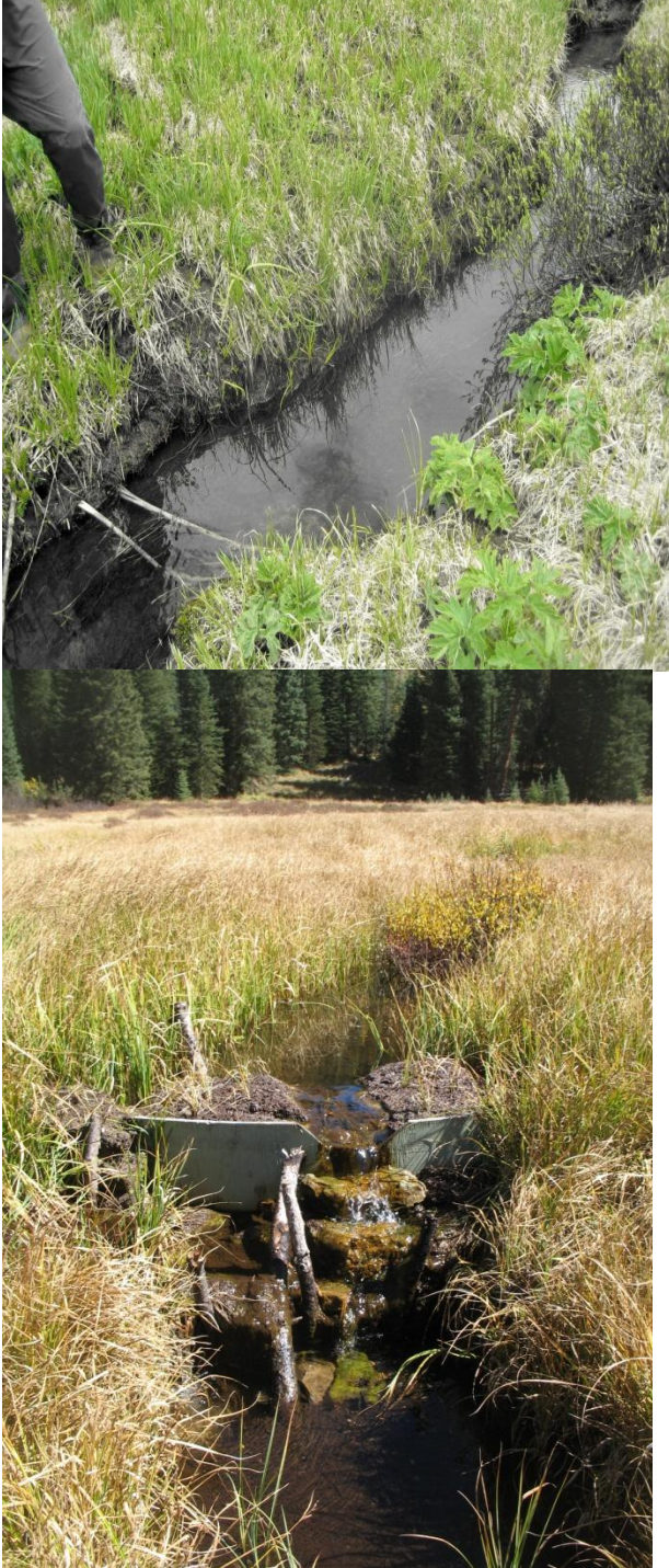
Figure 8. Pre restoration (left) and post restoration (right) view of plywood dam in Lateral Moraine Fen. Dam has v-notched weir, rock armoring on spillway, and has been filled with peat blocks planted with sedge plugs.
