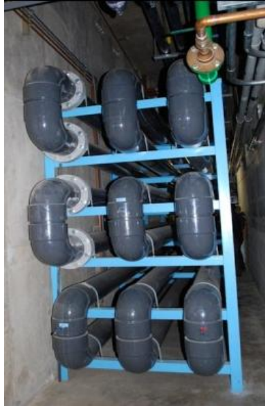
Figure 3.1. Pilot pipe-loop facility at Fort Collins Municipal Water Treatment Facility.
