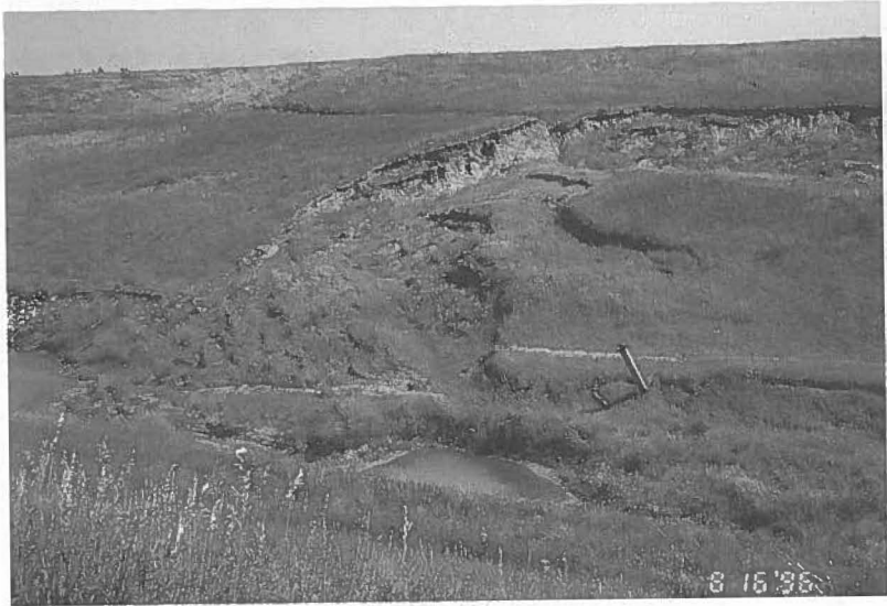
Fig. 3. This is an example of some of the severe deep slides which have occurred on the McClusky Canal (note movement of pipe at mid right of picture)
