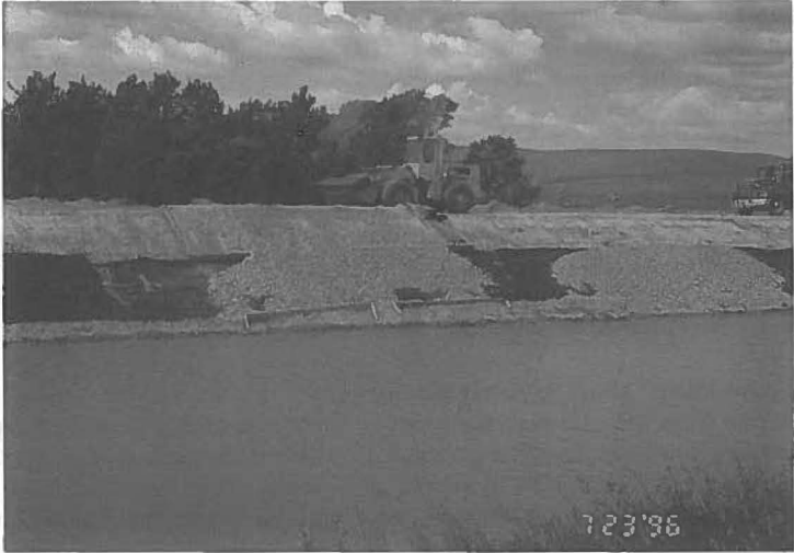
Fig. 11. The beach belting material being placed on the geotextile on the canal bank.
