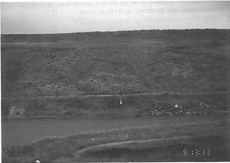
Fig. 2. The two slides in the center and right side of the picture are examples of shallow slides which have occurred on the McClusky Canal.
