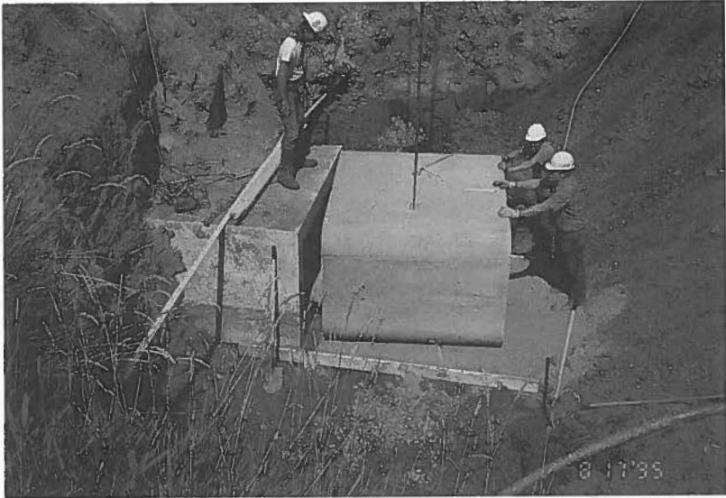
Fig. 5. Placement of box culvert to repair slide area where right-of-way width was limited.
