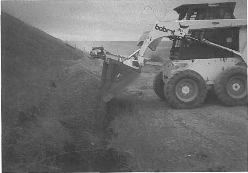
Fig. 7. V drain installation at the outside of the O&M road. Note the drain tubing at the bottom center of the picture.
