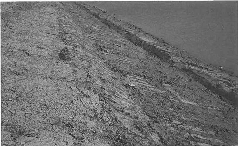
Fig. 10. Organic and other foreign material is removed followed by placement of material on the bank. The bank is then smoothed, compacted and a keyway (upper right) installed to prevent slippage of material.
