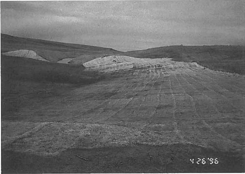
Fig. 6. An overall view of the completed work shown in Fig. 5. The area has been seeded and a mat installed to prevent erosion.
