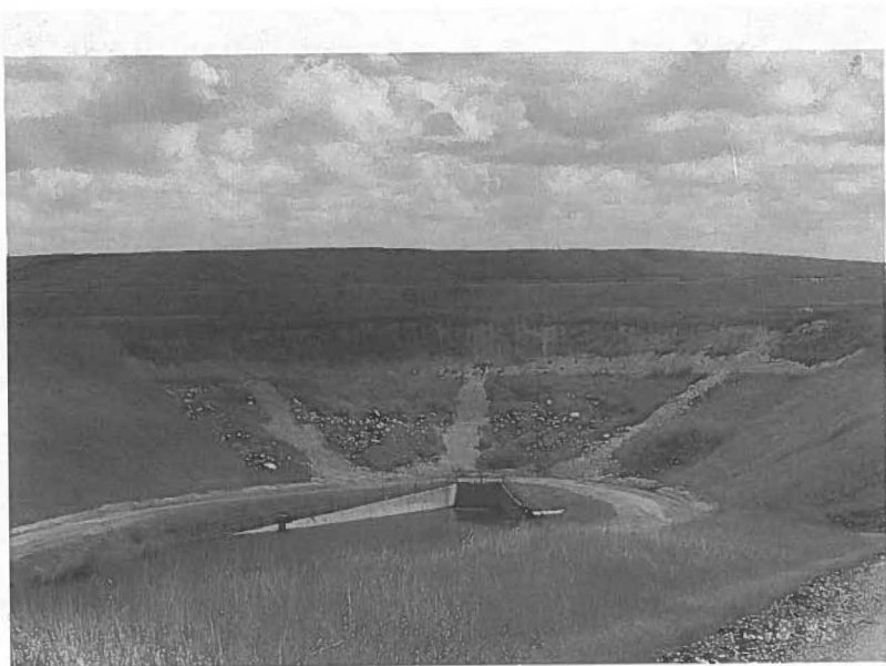
Fig. 4. Completed french drain work on a slide which jeopardized a state highway and railroad track above the slide.
