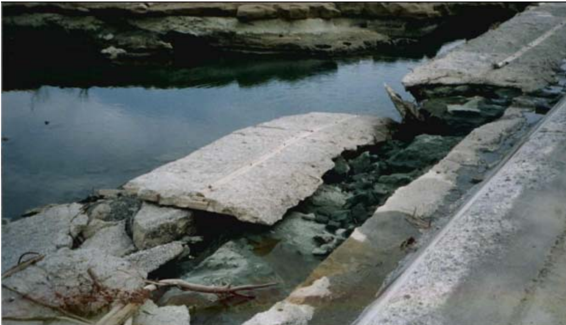
Figure 4. Partial failure of apron of Capay Diversion Dam in 2003
