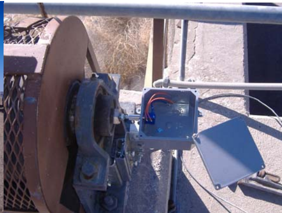
Figure 6. Gate Shaft Monitor
