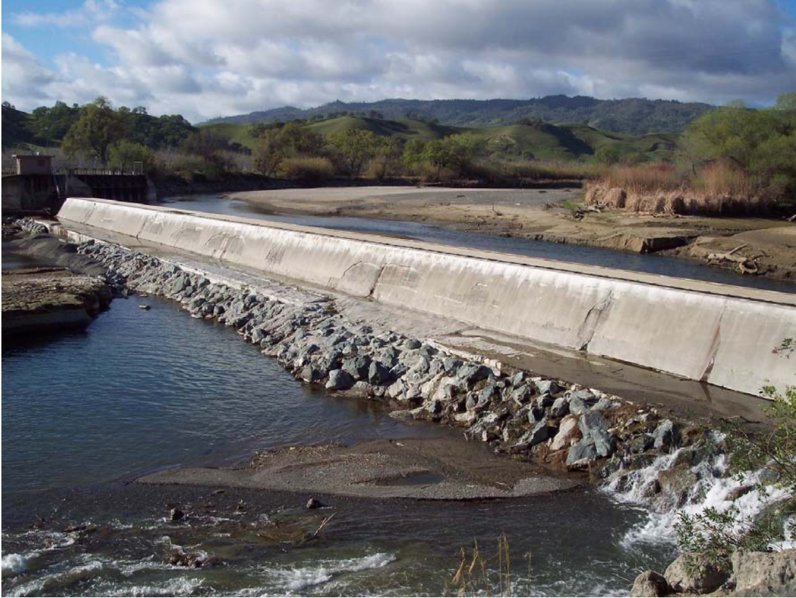
Figure 3. Photo of Capay Diversion Dam showing Cache Creek streambed degradation and local scour at end of apron
