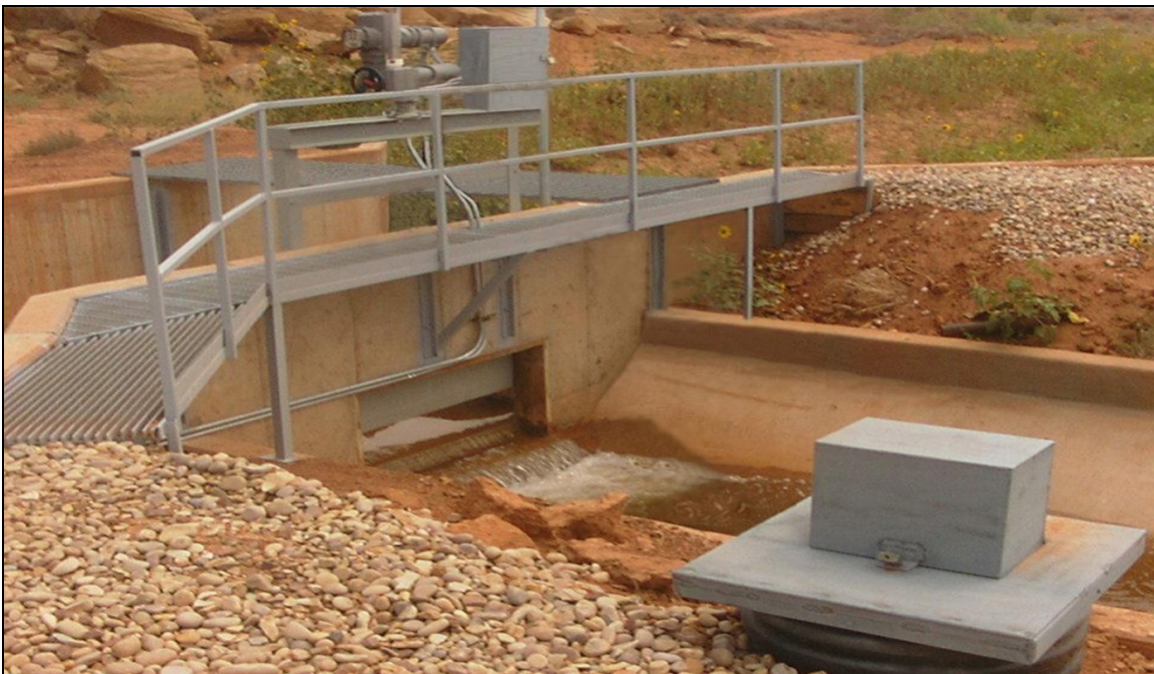
Figure 3. Inlet Pond Automated Gate
