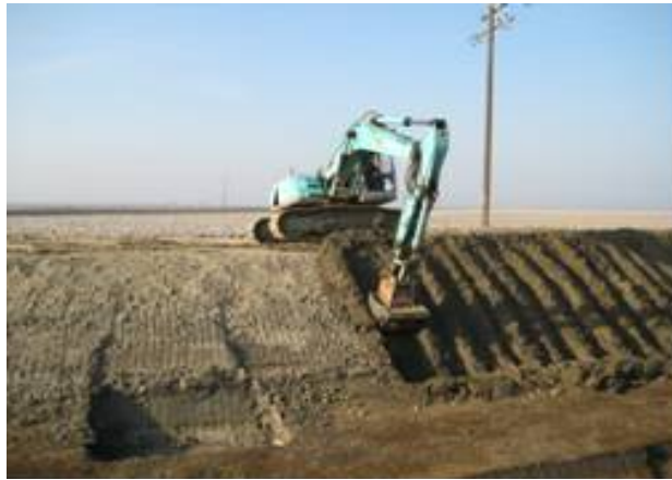
Figure 8. Compacting the canal banks on the James ID main canal with an MBW vibratory roller
