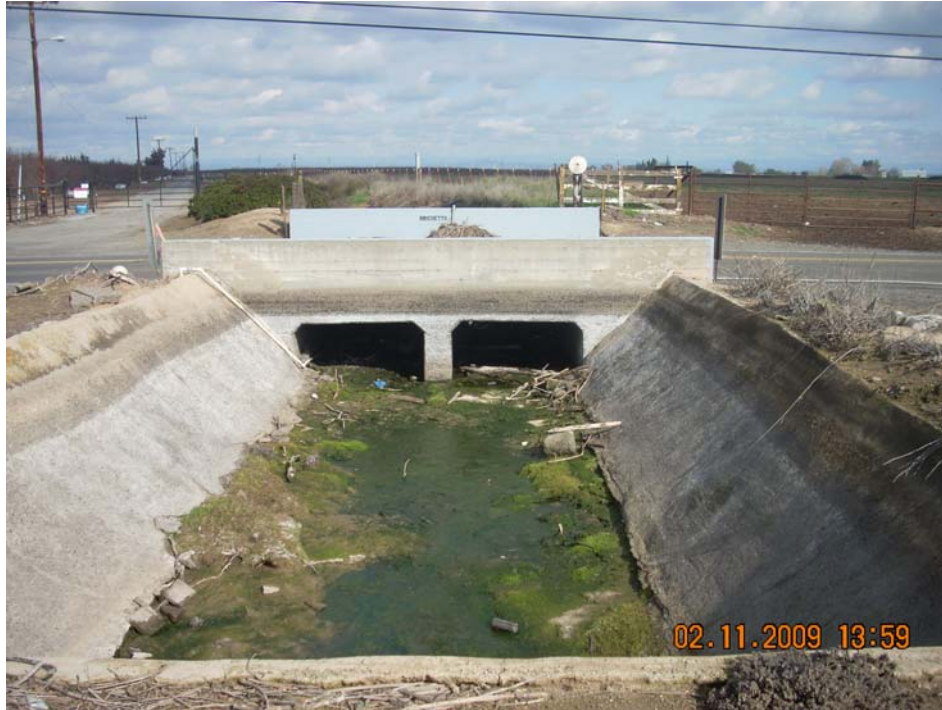
Figure 3. OID Brichetto Lateral Conduit Crossing at Oakdale Waterford Highway
