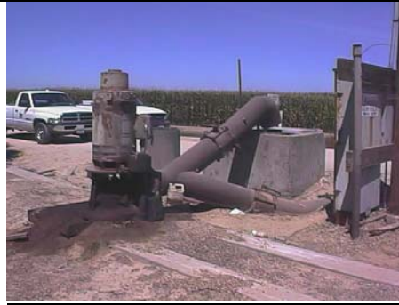
Type of Facility: Irrigation Pump No. of ID's: 238 Total Acres: 89,911
