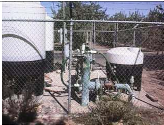
Type of Facility: Pump and Micro Irrigation System No. of ID's: 1 Total Acres: 56
