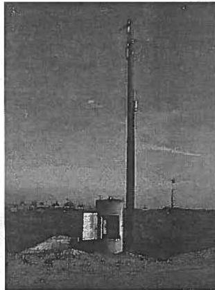
Figure 7 - Remote SCADA site
