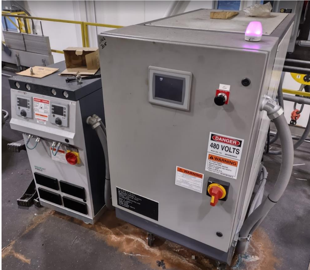
Figure 11: Hot water unit (left) and jet cool unit (right) in production (photo permission from Mercury Marine)
