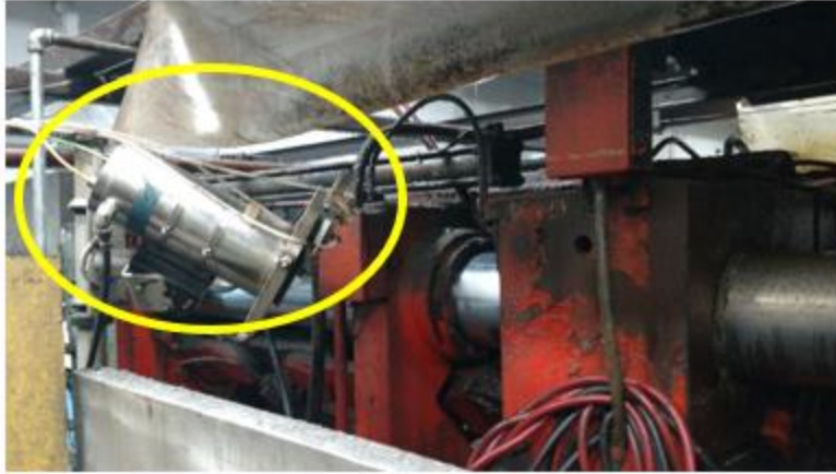
Figure 79: Thermal image camera system install on die cast machine [45]
