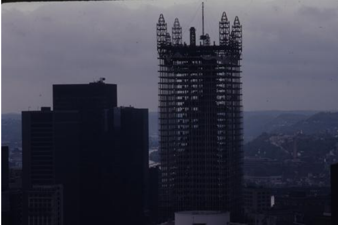
Figure 34: The construction of the Pittsburgh Plate Glass building in 1981, the building is seen as a symbol of Pittsburgh's turn around in a new modern era.
