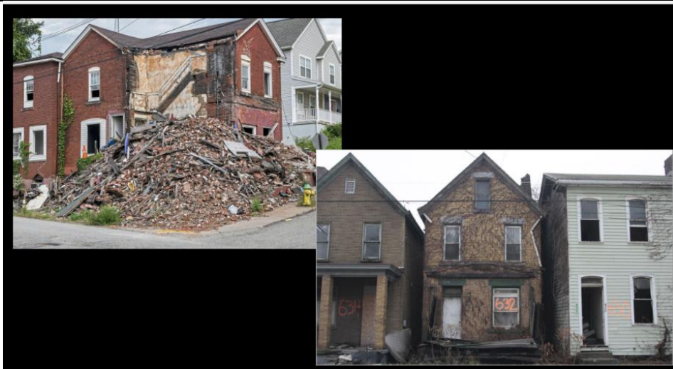
Figure 35: the beginning of the destruction of the Homestead Mill; Figure 36: abandoned worker homes in McKeesport; Figure 37: Dilapidated buildings in Braddock; Figure 38: abandoned homes in McKeesport. Photos retrieved from google image search
