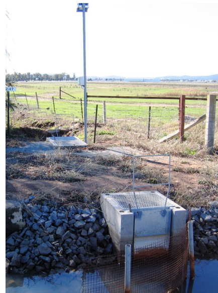
Figure 8. Doppler Meter - Transducer (left) and Turnout Emplacement (right)
