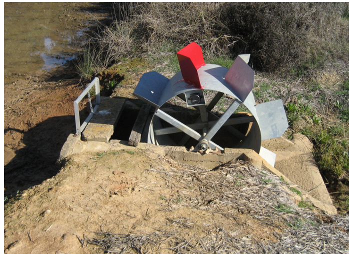
Figure 7. Dethridge Wheel Farm Turnout Meter – Goulburn-Murray Irrigation District
