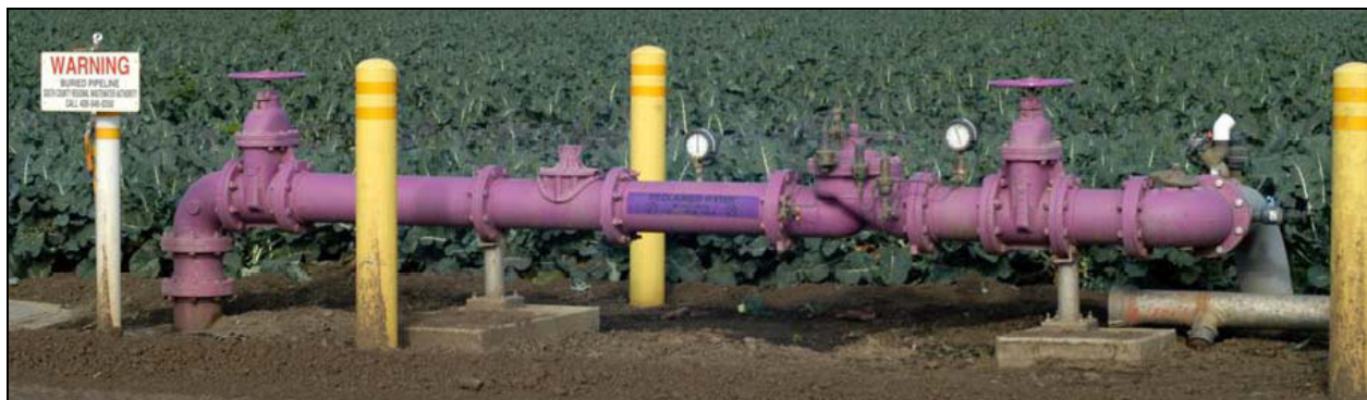
Figure 6. Irrigation Turnout on the South Pipeline
