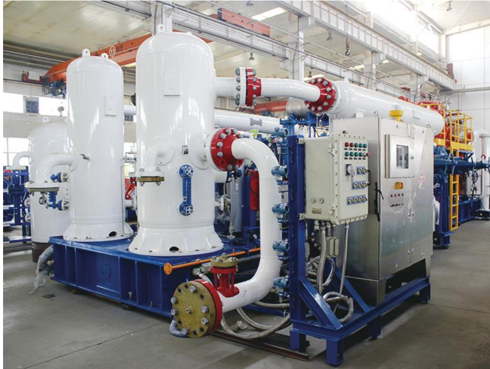
Figure 2-4: Interior View of a Natural Gas Compressor Station (source: http://go.jereh.com )
