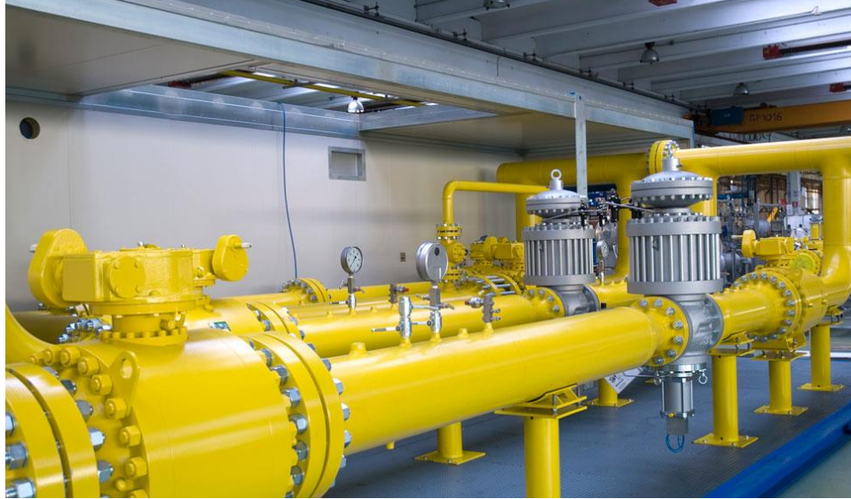
Figure 2-5: Natural Gas City Gate Station (source: https://www.fiorentini.com )
