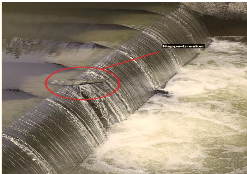
Figure 6. Aeration of the water nappe by the nappe-breakers for relatively low flow regime (Gate A, Flow Rate <math>< 50 \text{ ft}^3/\text{s}</math>).
