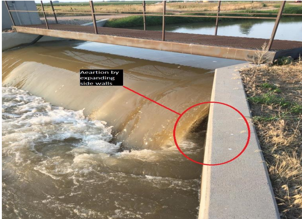
Figure 7. Aeration of the water nappe by the expanding side walls for relatively high flow regime (Gate A, Flow Rate > 50 ft 3 /s).
