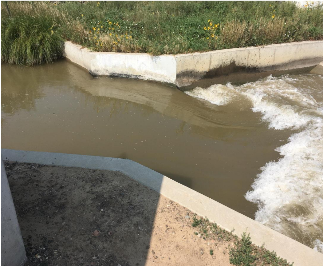
Figure 42. Flow over Gate C, indicating inadequate nappe aeration.
