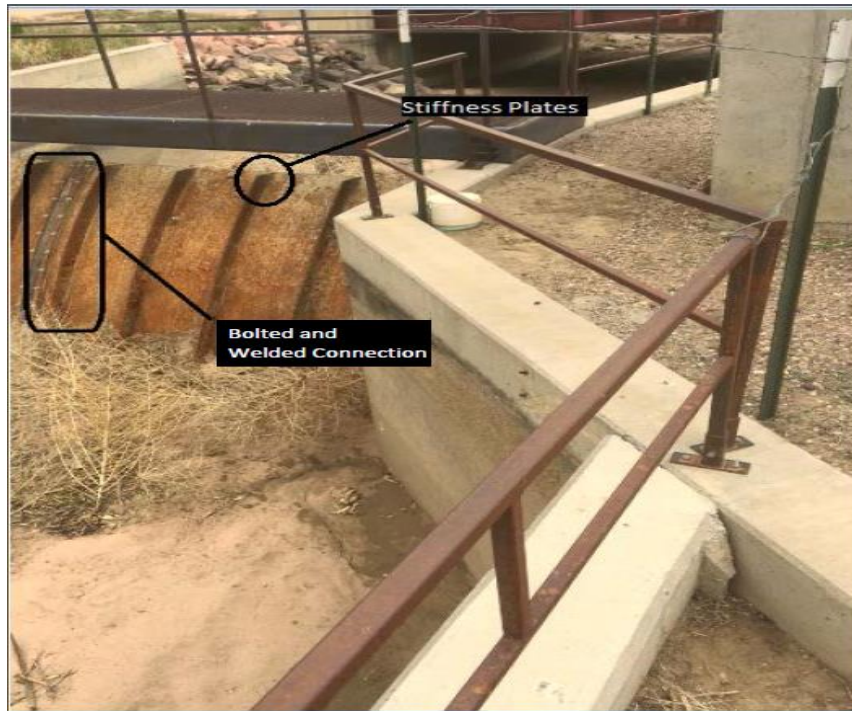
Figure 5. Rigid connection between the gate leaves, and stiffness plates (GateA).
