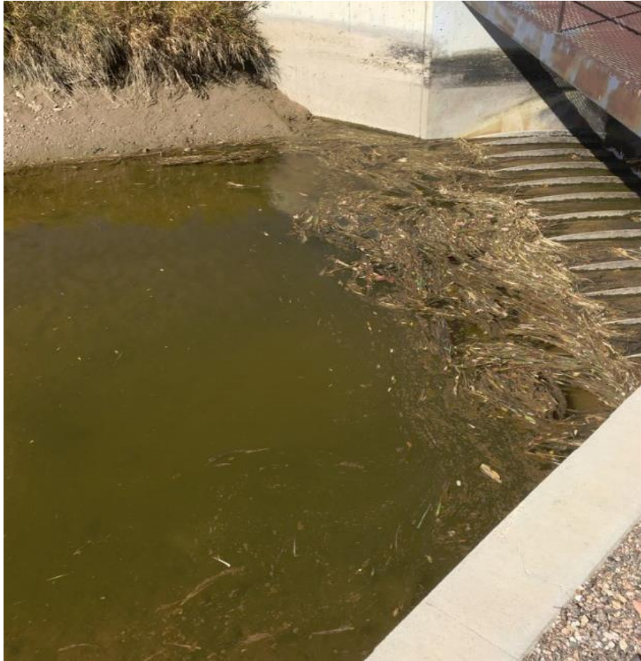
Figure 53. Sediment Load and Debris Accumulation under the low flow effect in the canal
