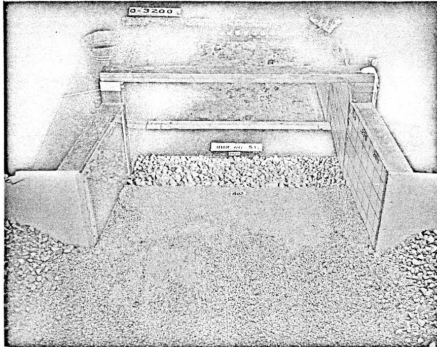
Fig. 35 Protection of discharge channel bed for total length of 35 meters beyond end sill.
