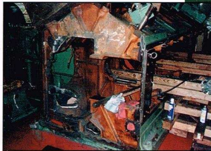
Lower right: Frame ready to receive fabrication and new main bearing saddle.
